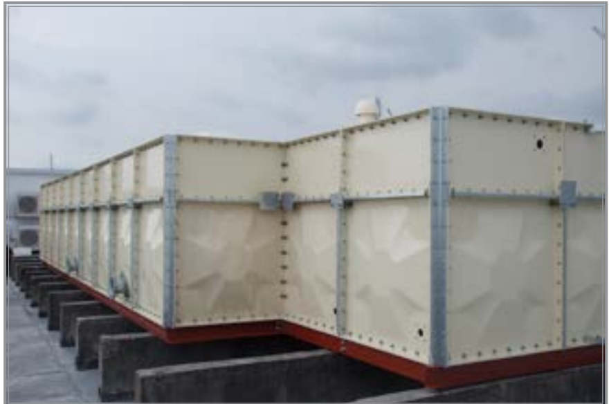
An installed FRP tank
